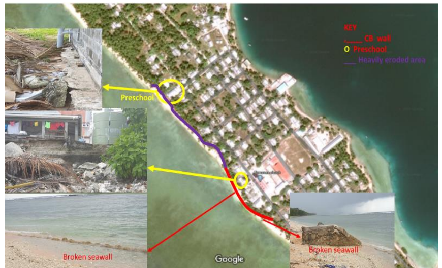
Figure 3: Heavily eroded area, Nanumea 27 July 2020
